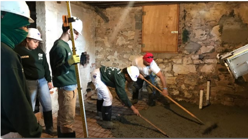
Carpentry students learned to pull and spread a concrete floor, a challenging task!
