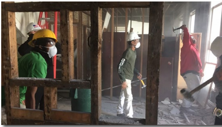
It was all hands on deck for demolition at the Michelle House in New Haven.
